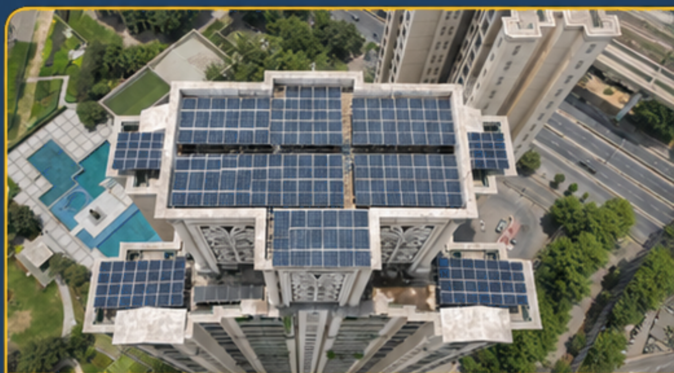
Structured rooftop deployment
