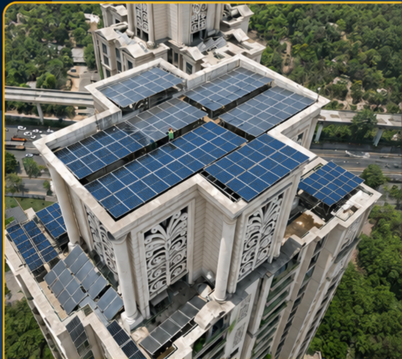
High-rise rooftop solar installation
